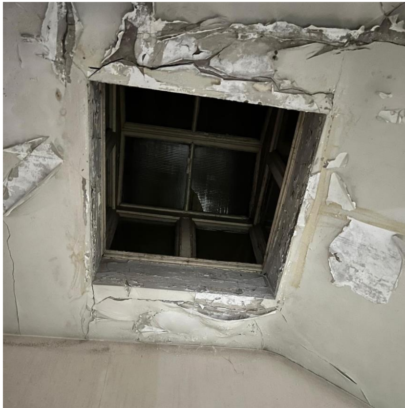
Figure 48 – Photograph of inside of existing roof lantern. The lantern has been made weathertight and boarded up whilst the application is considered.
